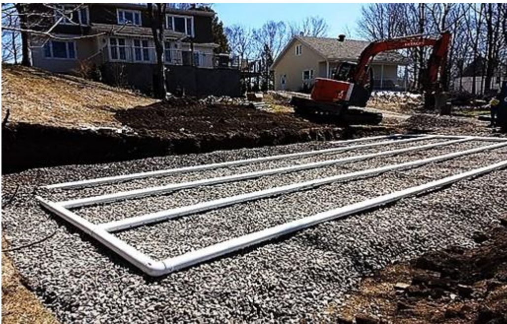
Fig. 35. A drainfield being installed, with many thanks to the author Nonztp and Wikipedia.
